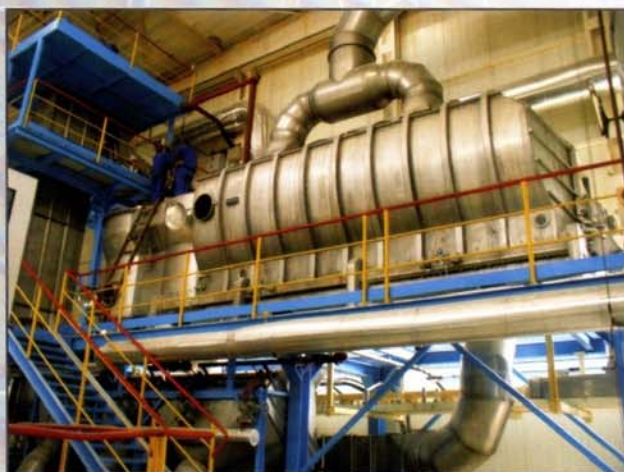
Assembling of the installation for drying and cooling of sugar in the sugar Factory Kruszwica S.A. (KSC Polski Cukier). The installation was started up in 2006, capacity 50 t/hr.
