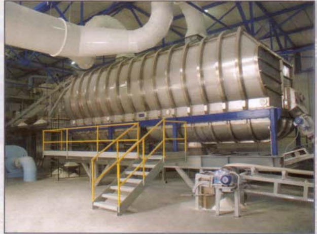
Fluid bed cooler installed in 2004 in the sugar Factory Maloszyn S.A., capacity 800 t/day. In 2006 the cooler was reallocated to the sugar Factory Strzelin S.A. (Südzucker).
