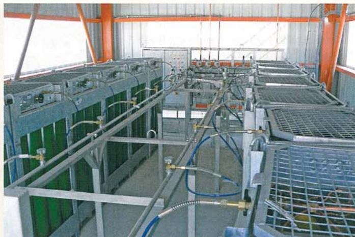
Fig. 3: Batteries of high pressure N 2 packs
